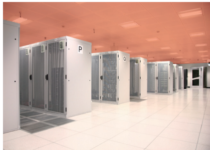
Ceiling protection at Data center
